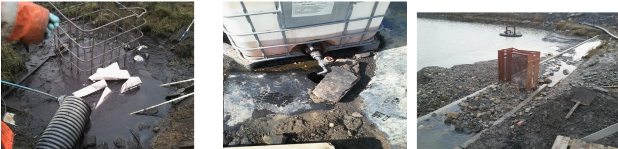
Alum blocks tipped into waste stream, Aluminium liquid cracked valve & empty Alum basket
